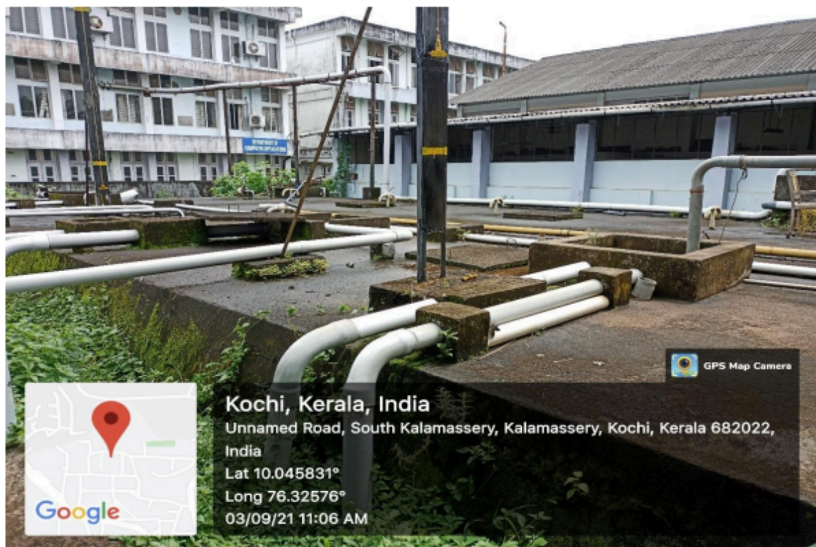
Fig. 14.5.22. Maintenance of waterbodies and distribution system at CUSAT campus
