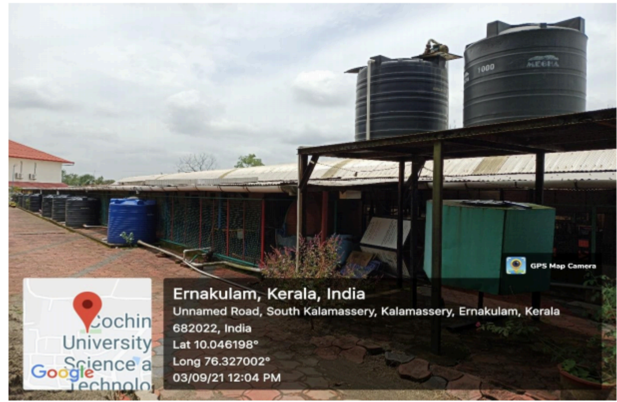
Fig. 14.5.21. Waste water recycling plant at CUSAT
